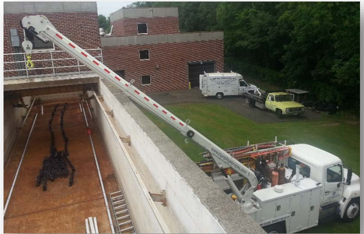
Pumping Services, Inc. installation and service group recently completed a retrofit of a Polychem chain and flight system at a Waste Water Treatment Facility
