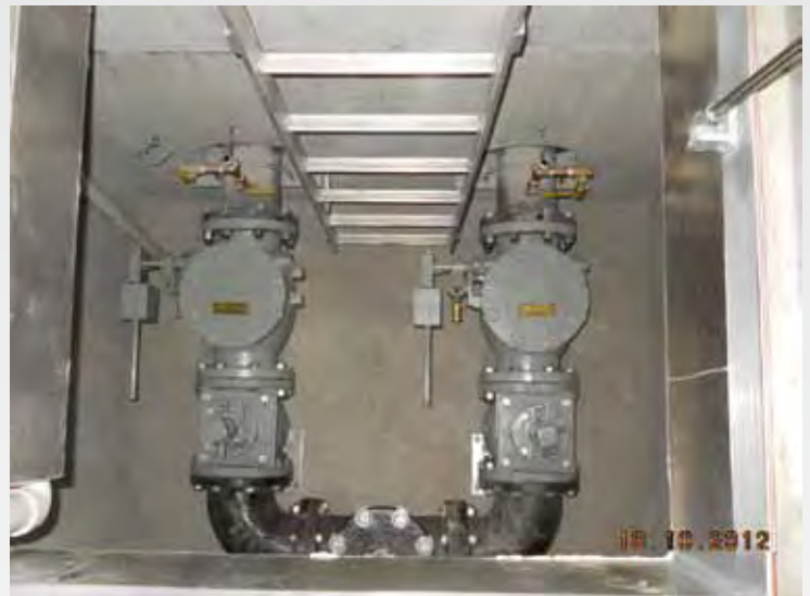
Valve Assembly in Valve Vault, pre-assembled in factory.
