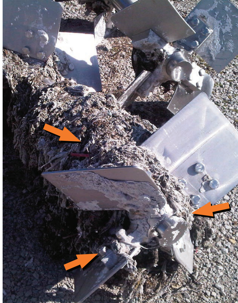
Rag buildup from competitor installation
