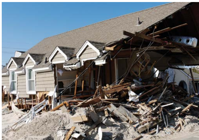
Destruction from Superstorm Sandy in Mantoloking, NJ.
