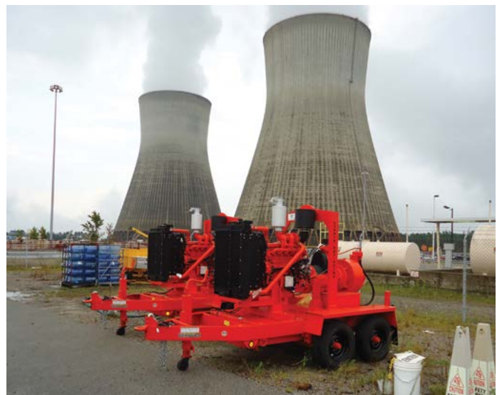
Godwin pumps positioned in front of cooling towers.
