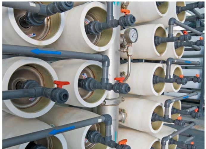
Racks of filters in a desalination plant.
