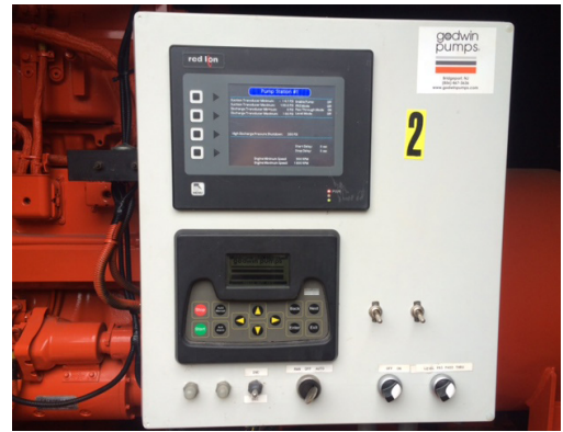
Xylem customized the Advanced PrimeGuard Controller to address multiple customer requirements, including a tie-in to the HRSD network SCADA system.
